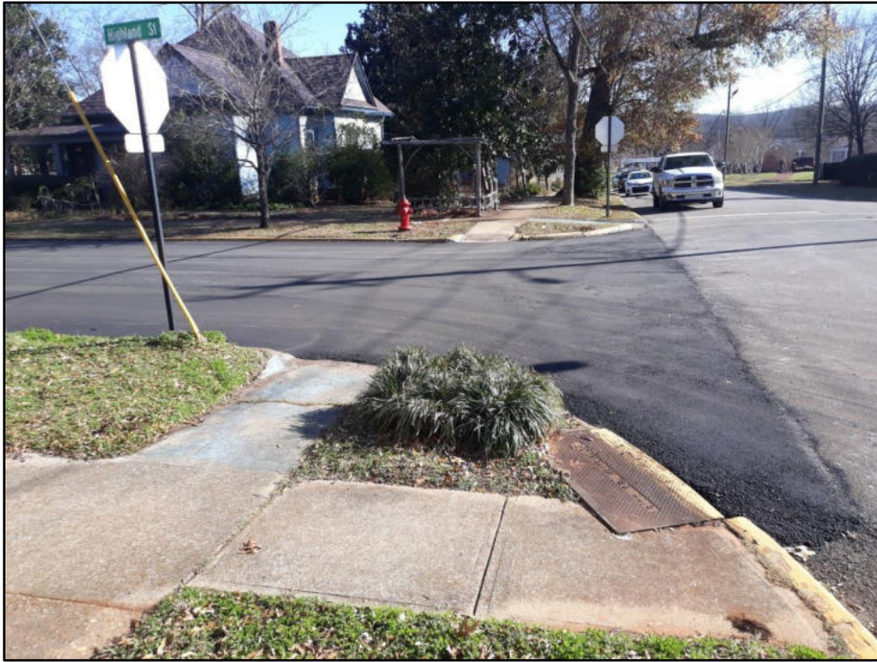
74 – Bloch St at Highland Two older style curb ramps need updating, lacking curb ramp in one direction
