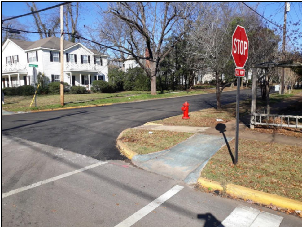
74 – Bloch St at Highland Older style curb ramps need updating
