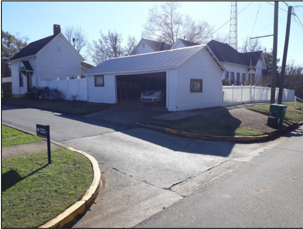
61 - Valley St from Vine to N Boundary Need 3 curb ramps installed on this block, 1 of which at alley currently has 2 steps
