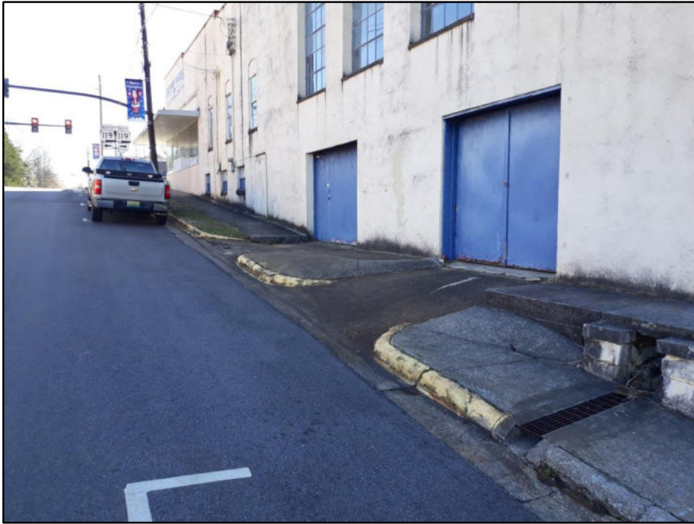
50 – Shelby St from Main to Valley Non-compliant sidewalk across several driveways, difficult grades to correct
