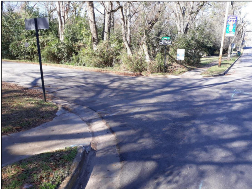
8 – Middle St at Alabama Has 4 outdated curb ramps that lack detectable warnings and have cross slopes >2%
