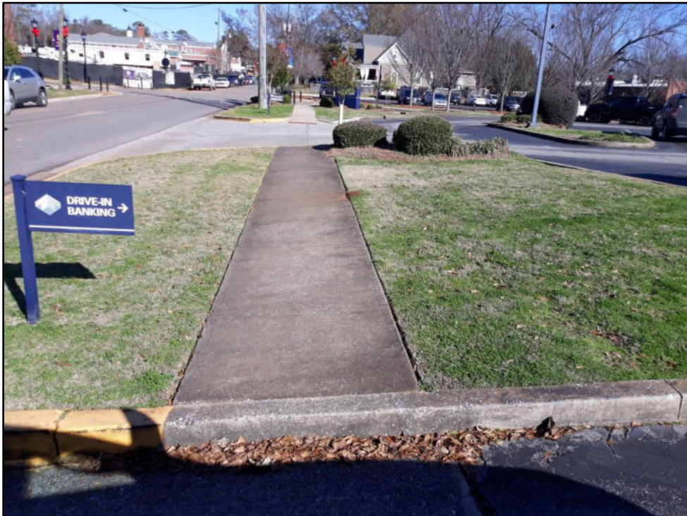
61 - Valley St from Vine to N Boundary Need 3 curb ramps installed on this block, 1 of which at alley currently has 2 steps
