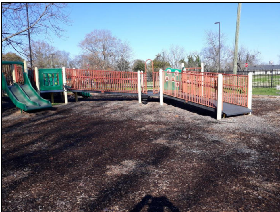
E – Dailey Park Playground equipment is designed to be ADA accessible, but the ADA access is 6" off ground
