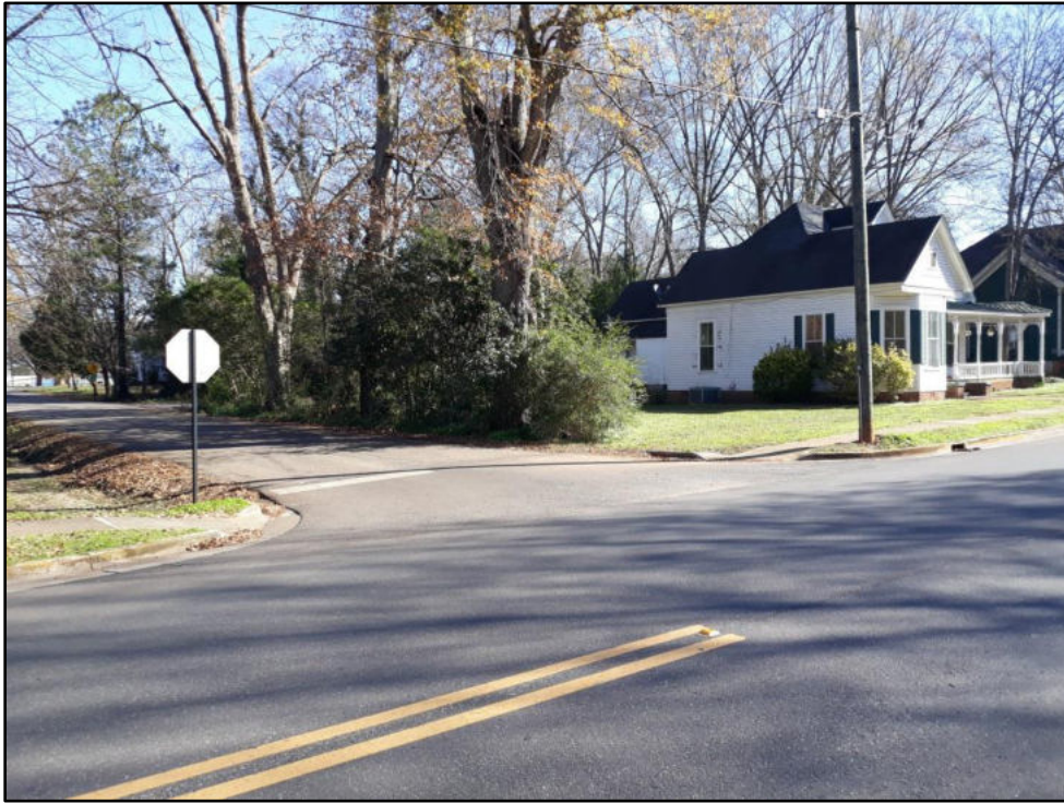
8 – Middle St at Alabama Has 4 outdated curb ramps that lack detectable warnings and have cross slopes >2%
