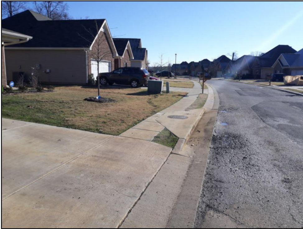
A – Moores Spring Road in Amersee Lakes Subdivision 2500 LF of 3' wide sidewalks, cross slopes exceed 2% at some driveways
