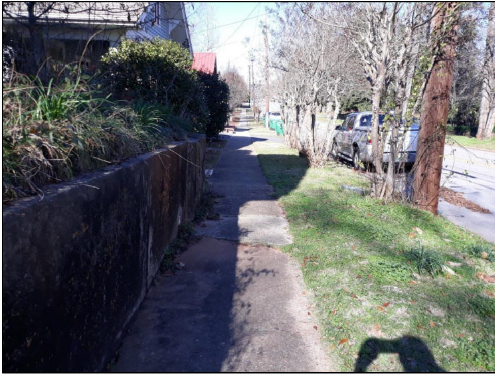
1 – Shelby St between E Boundary and Alabama Older sidewalk with some disjointed panels, width less than 48”
