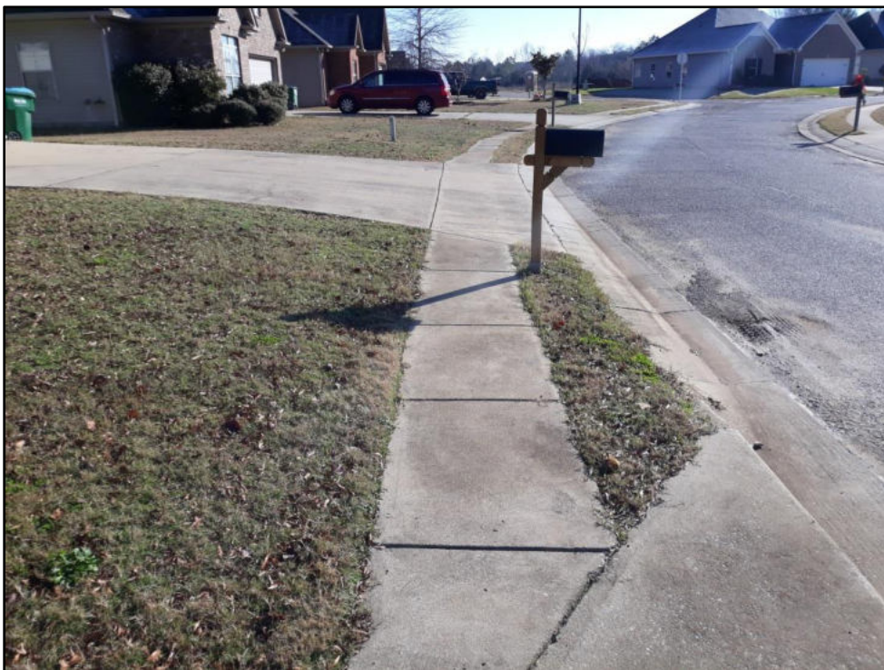
A – Moores Spring Road in Amersee Lakes Subdivision 2500 LF of 3' wide sidewalks, cross slopes exceed 2% at some driveways
