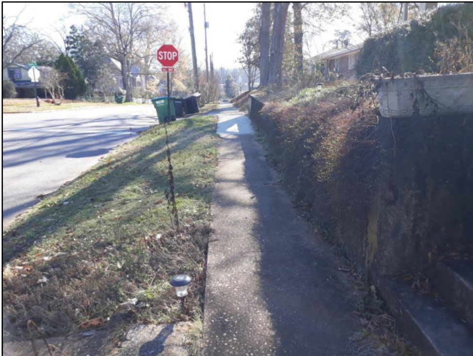
2 – Shelby St between E Boundary and Alabama, south side Older sidewalk with some disjointed panels, width less than 48”
