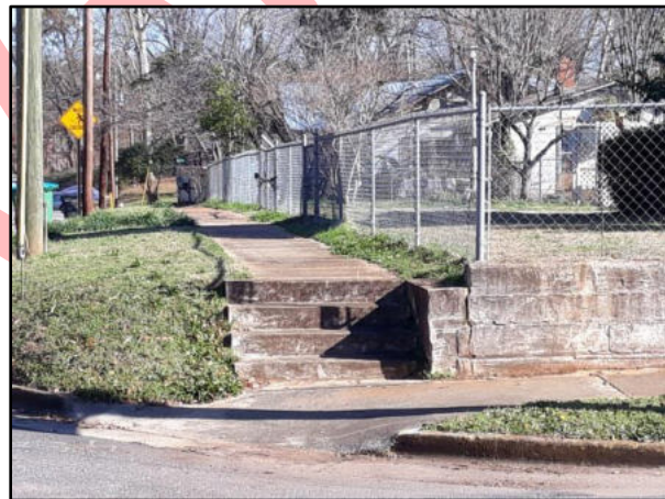
Fig. 9 – Older non-compliant curb ramp on Middle St
