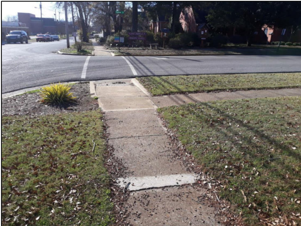
73 - Oak St at Plowman Updated curb ramps and sidewalk tie ins, also has had grinding to remove discontinuity
